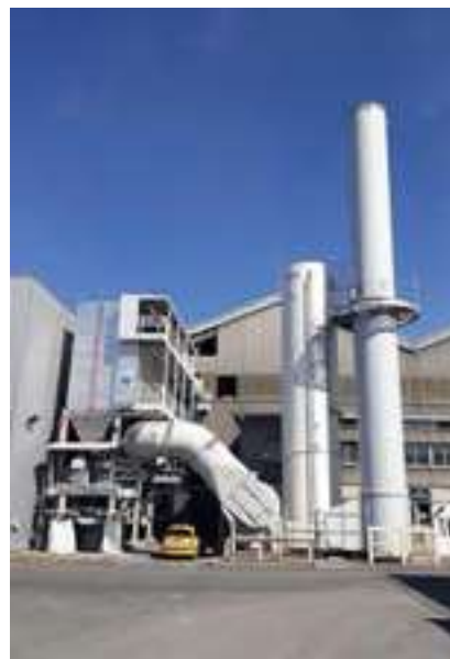
The Issoire plant’s project is expected to recuperate heat from the furnace exhaust fumes to provide a new source of heat for municipal facilities
