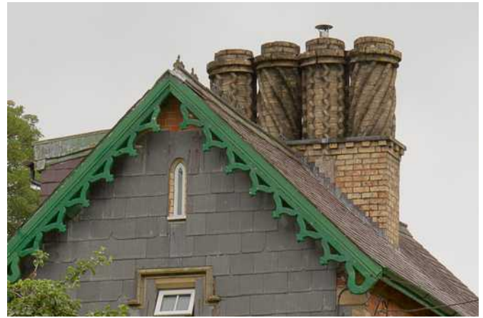
Bricks as an architectural feature on chimneys. Penygreen Lane, Llanidloes. Photo ©Richard Becker.
