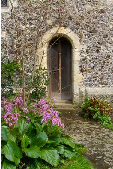
Flint wall with Caen stone doorway. St Peter's Church, East Blatchington, Sussex.
