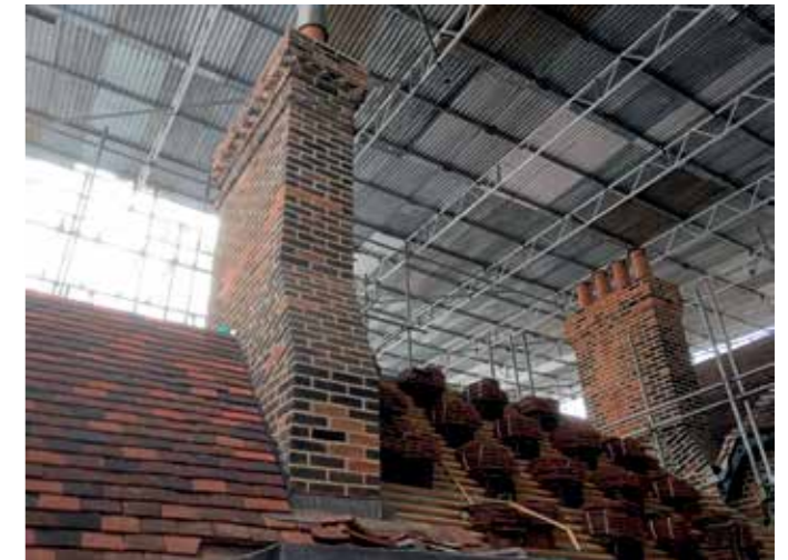
■ The same chimney following partial reconstruction and repair with roof tiling work ongoing. Note the reinstated chimney pots to the stack on the right.
