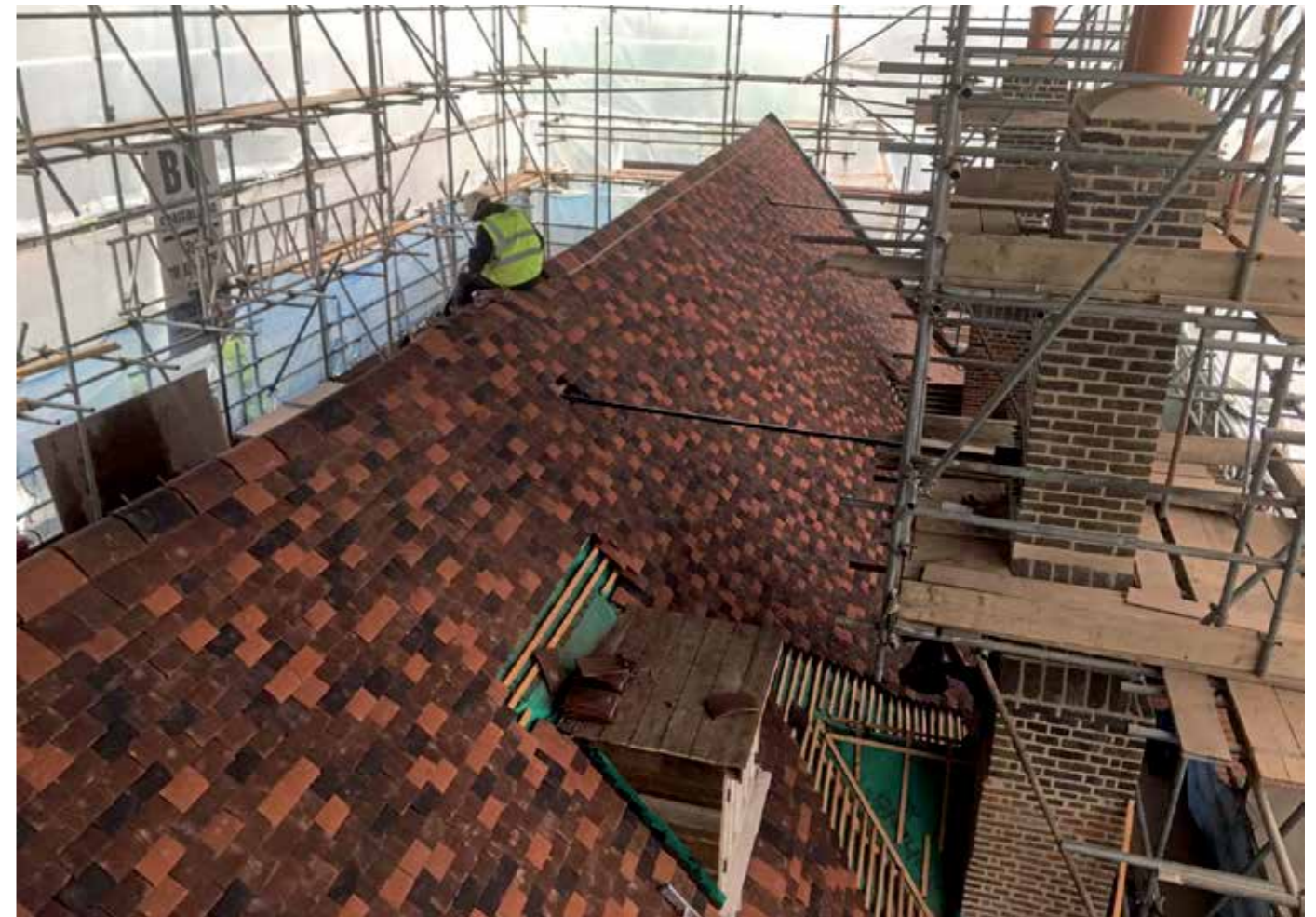
■ The near-complete library roof, with the repaired and reinforced tall chimneys on the right. The roofing is a mix of three colours of hand-made plain clay tile made in Kent.
