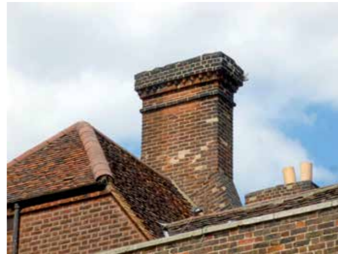
■ A closer view shows the badly weathered condition of chimney stacks.
