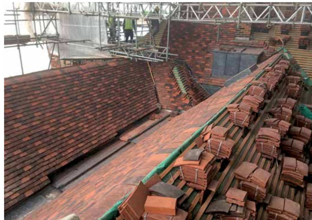
■ The near complete roof above the bursary with new handmade roof tiles stacked out awaiting installation.
