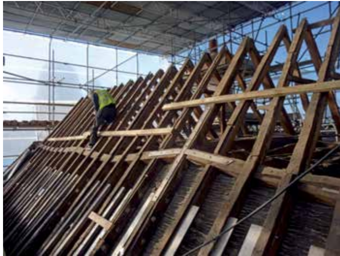
■ Timber repairs underway on the 1620s library roof. Having been reinforced with stainless steel brackets to secure the roof more firmly to the walls, the historic structure now has many more years of useful service ahead of it.
