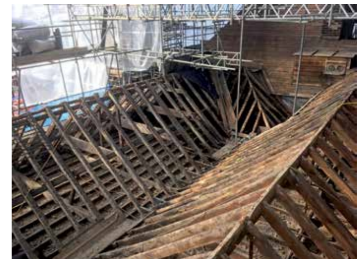
■ The same roof after removal of the coverings. Following clearance of debris from the left spaces, timber repairs were carried out and sheep's wool insulation installed.
