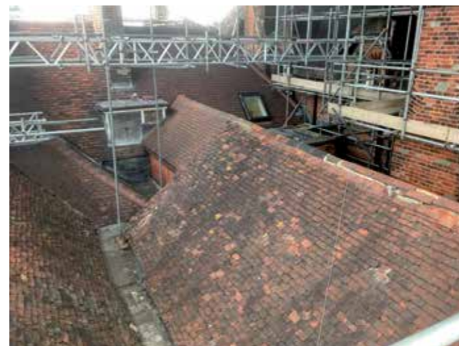
■ Roof coverings were all life-expired, in this case to the hidden valley over the bursary.
