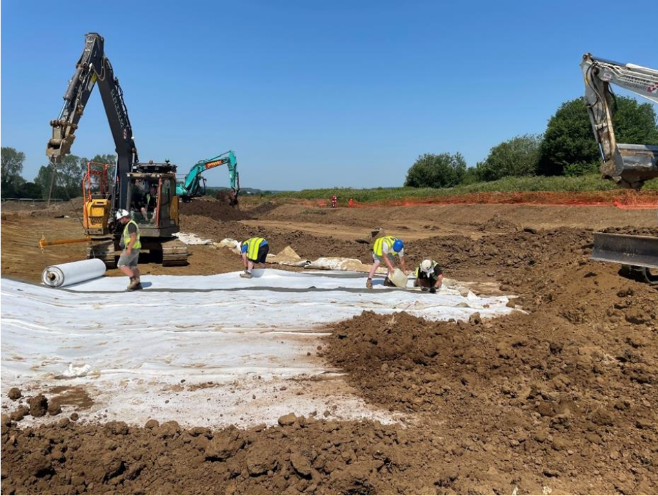
Figure 5.7. Example of GCL being laid out and covered by compacted soil. Photo courtesy of Water Design Engineers Ltd
