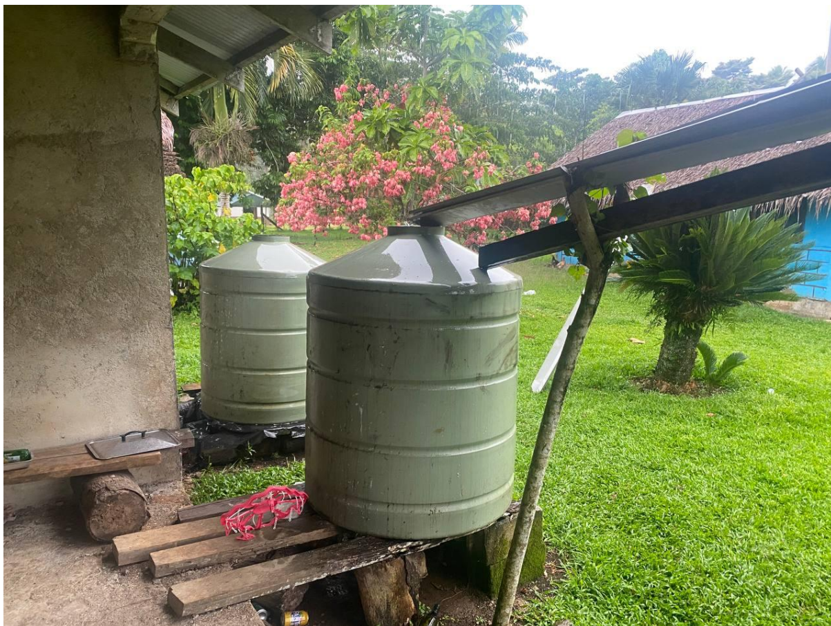
A water tank provided by the project to the family members
