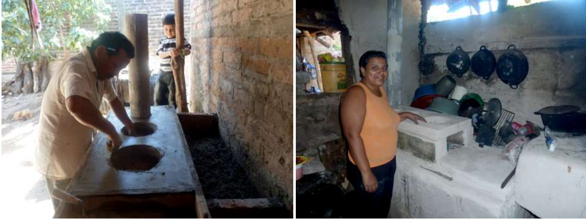
Above: New fuel-efficient cookstoves in construction (left) and a new stove in use (right).
