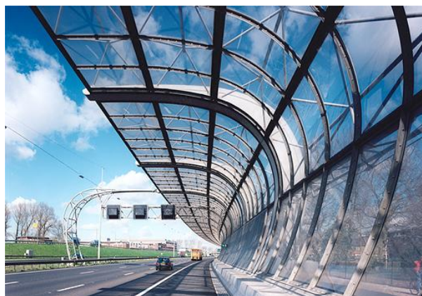
Figure 19. Barrier on the A16 Highway in the Netherlands
