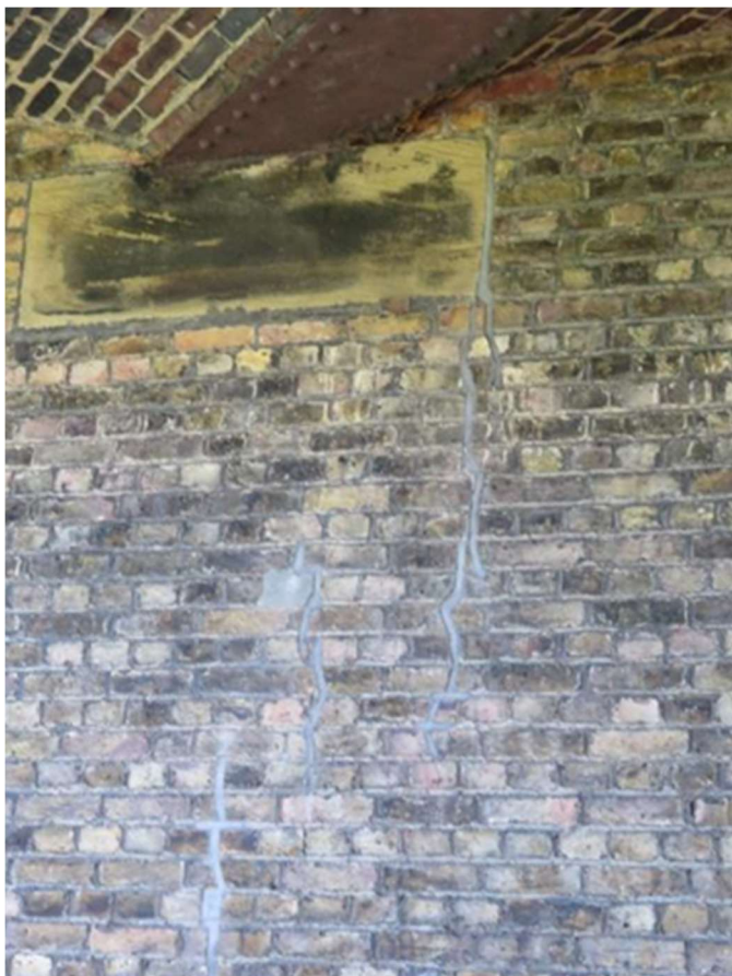
Fractures in abutment below padstone.
