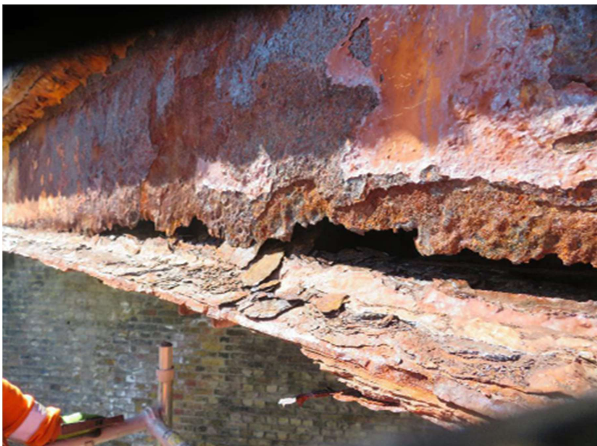
Southern edge beam severe corrosion.
