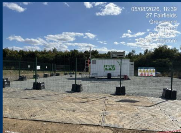
Hydrogen charging facility on site
