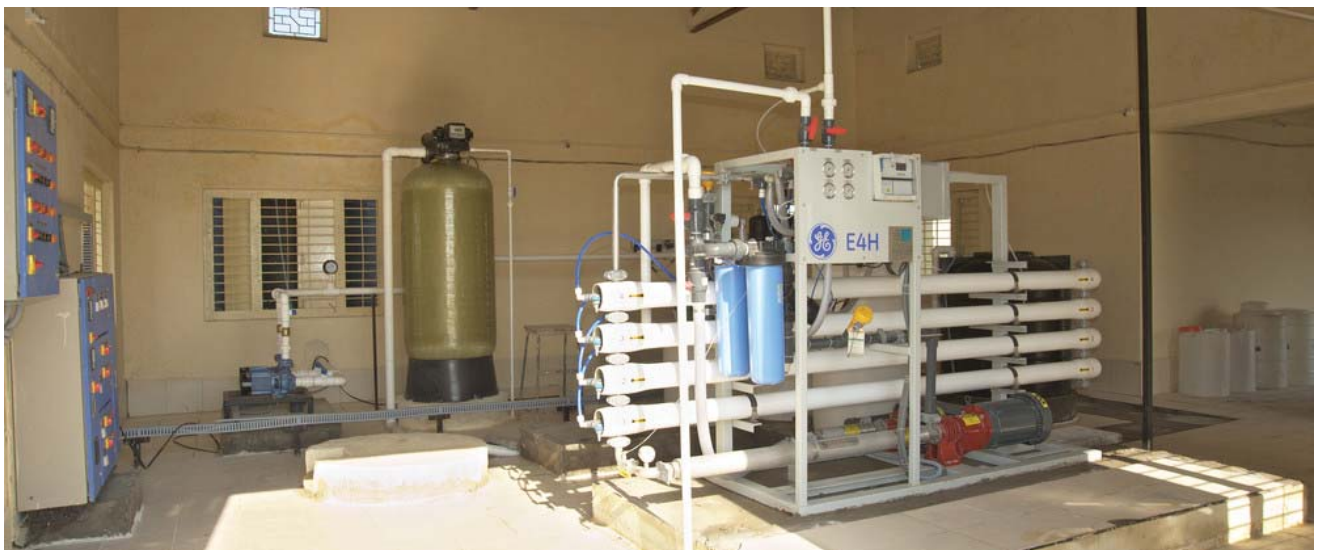
Reverse osmosis plant provides quality drinking water to communities in salinity affected coastal villages in Gujarat
