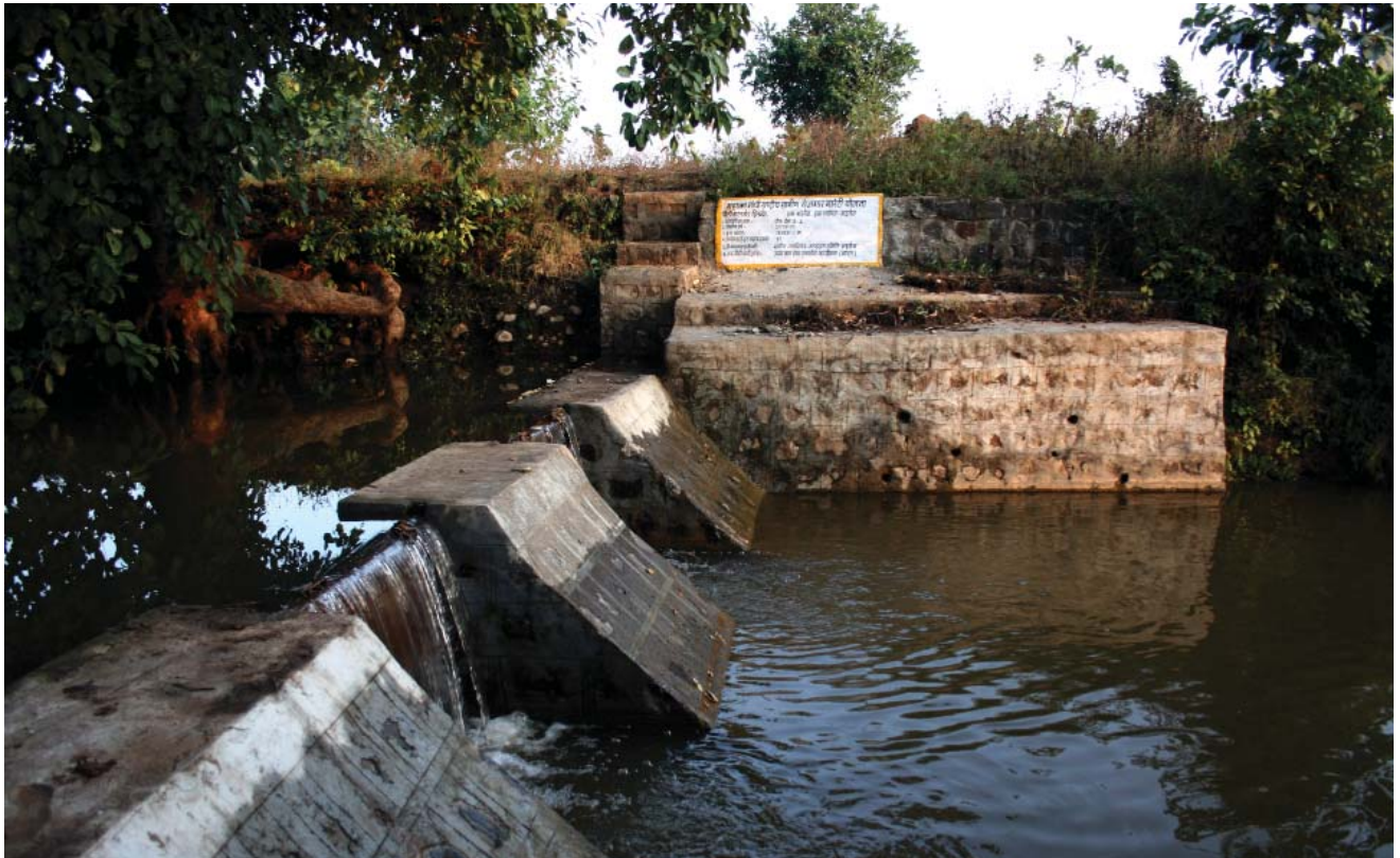
Assets such as this water harvesting structure constructed under MGNREGS have provided critical support irrigation and help recharge aquifers as well
