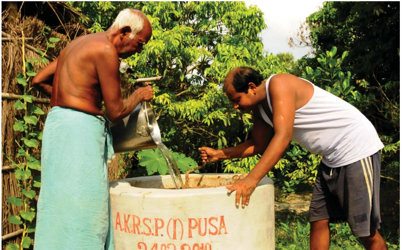
Biogas plant in operation in Bihar
